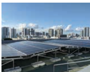
Solar panels on the rooftop of 202 Kallang Bahru
